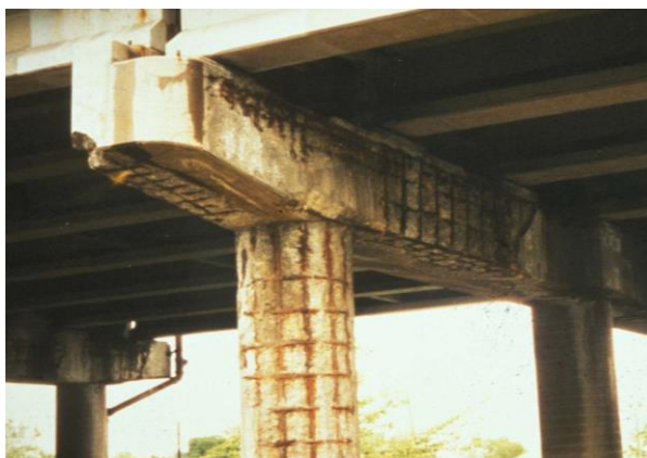
Fig. 1.1 Severely corroded reinforcing steel in this bridge column has resulted in spalling of the concrete cover and exposure of the steel reinforcement. (Ranger and Willams, 2011)[1]
