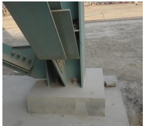
Fig 3: Cast-in L-Anchors supporting an industrial steel frame structure through base plate and pedestal arrangement.
