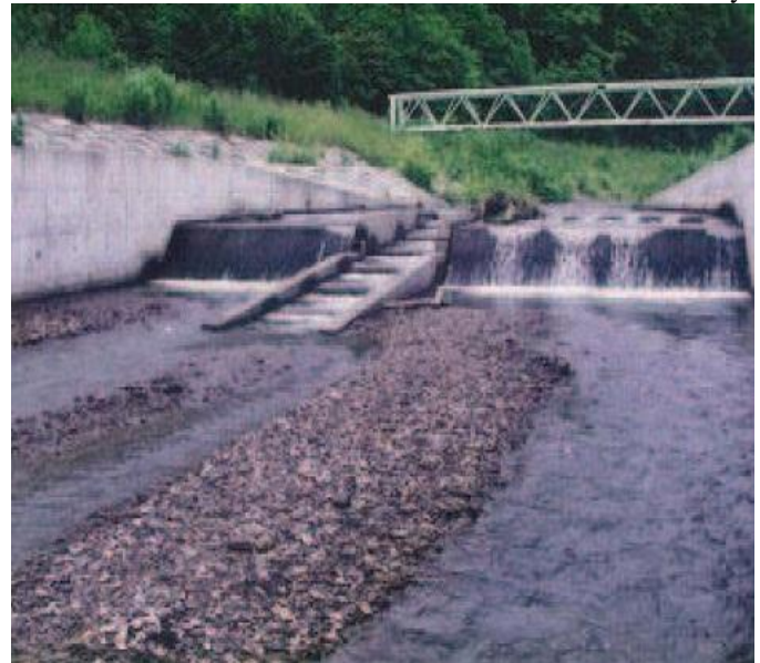
Figure 3: Improper flow conditions in low water condition at the downstream of the fish way
