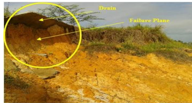
Fig. 1: Failure Plane beneath Slope Crest
