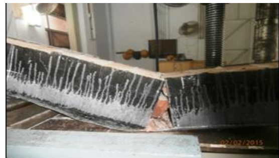
Fig.6: Failure mode of masonry beam
