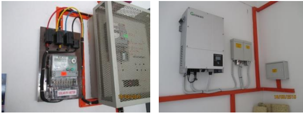
Figure 3: TNB solar electricity meter (L) to read the total PV yield distributed to the grid and the PV Inverter which converts the PV DC electricity current to AC current (R)
