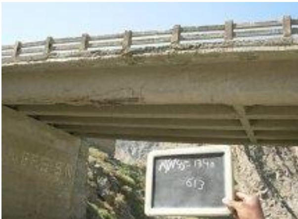
Figure 2 Damage to the Girder
