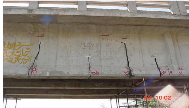
Figure 9 Cracks developed in the web
