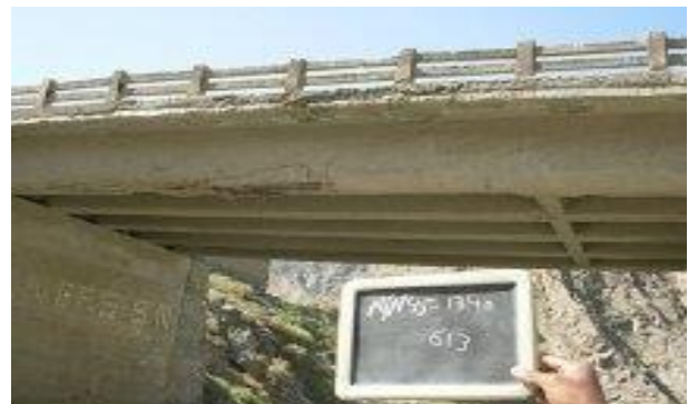
Figure 5 Damage to the Girder
