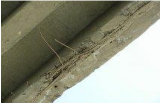
Figure 6 Pre-Stressing Strands Exposed
