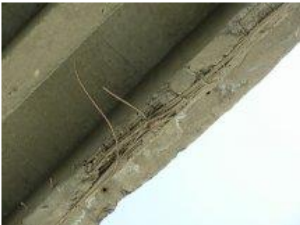
Figure 3 Pre-Stressed strands exposed
