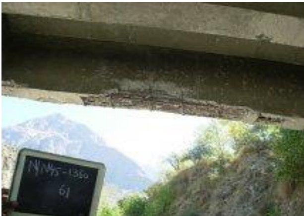
Figure 7 Damage to the Lower side
