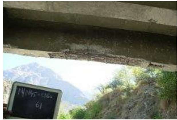
Figure 4 Concrete Deterioration in Girders
