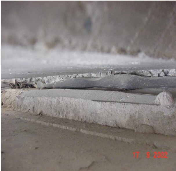
Figure 2 A view showing a failed elastomeric bearing pad observed in Sutlaj bridge
