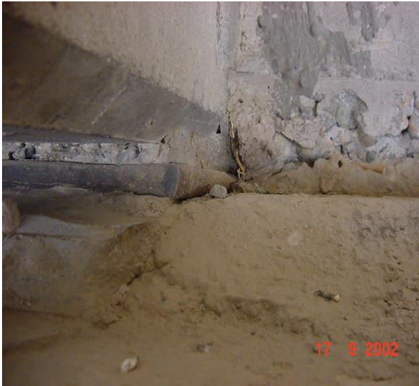
Figure 1 A view showing a failed elastomeric bearing pad observed in Sutlaj bridge
