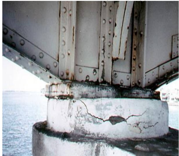
Figure 3 Failure of elastomeric bearing under Steel girders
