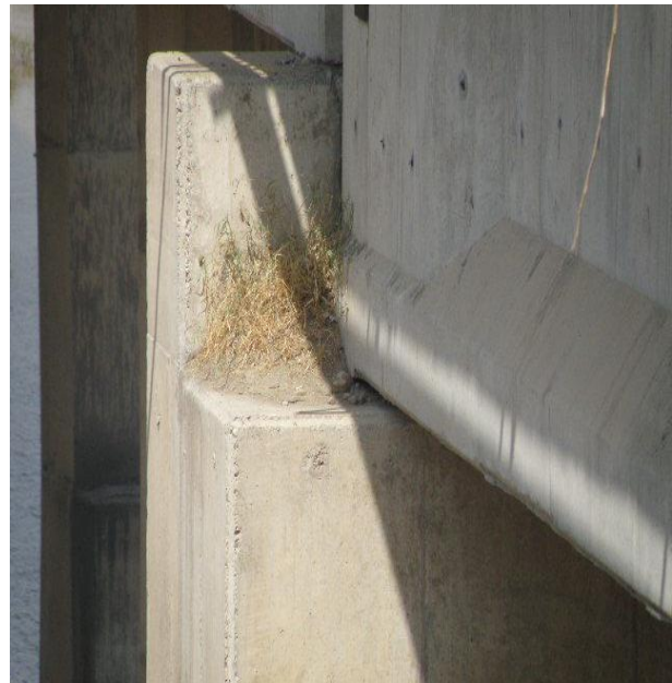
Figure 4 Vegetation near the bridge bearings at Kokbridge on Islamabad Highway
