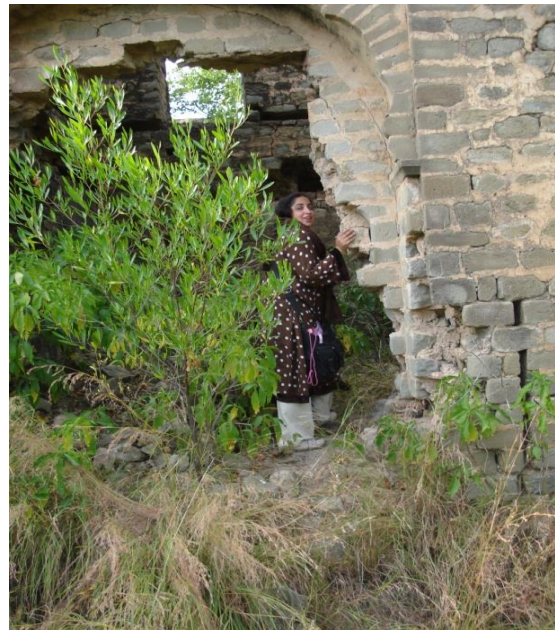
Fig. 7. broken Multifoiled arch of the elevation
