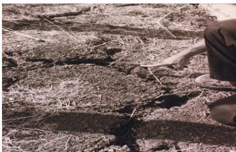
Fig. 3: This crack is at least 32 inches deep. The yardstick was easily inserted to this depth; narrower, less straight cracks may extend much deeper.
